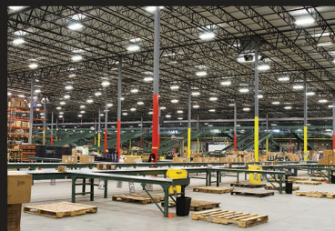
Energy Efficient Lighting
