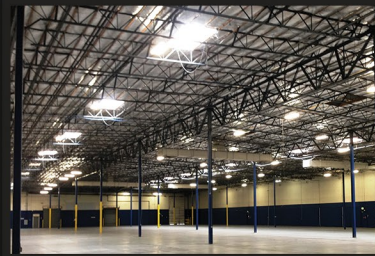
Energy Efficient Lighting
