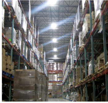
Energy Efficient Lighting
