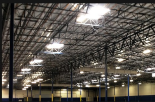
Energy Efficient Lighting
